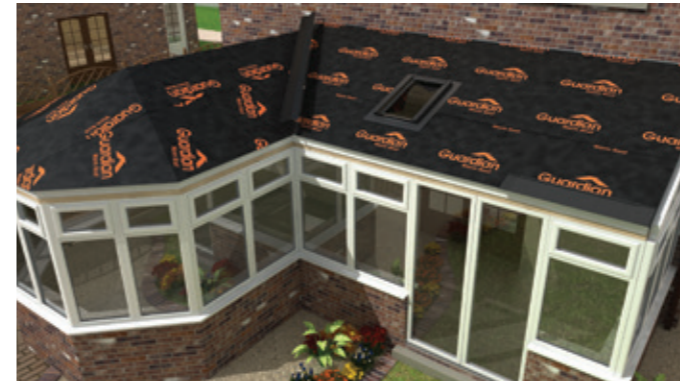
Breathable waterproof membrane is laid over the plywood and secured in place.
